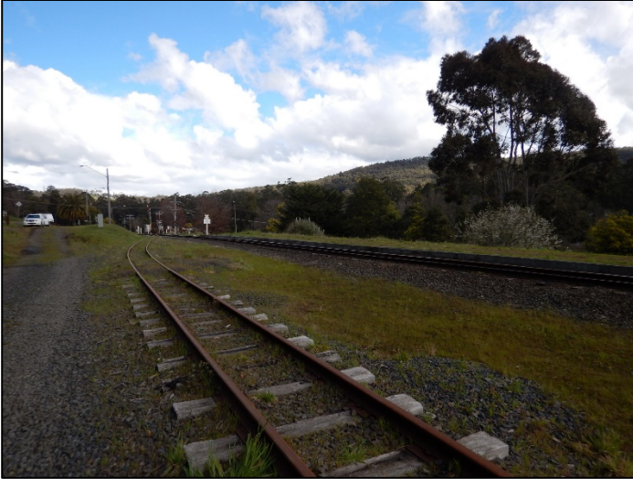
Plate 74 Grasses growing between ballast on the siding track (L. Tepper 4/9/17)
