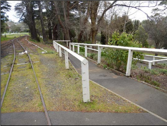
Plate 57 Ramp and siding to the west of the packing shed (L. Tepper 4/9/17)
