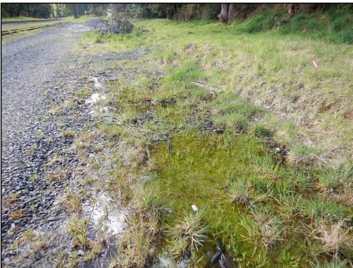
Plate 73 Areas of pooled water on the informal road (L. Tepper 4/9/17)
